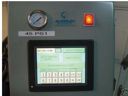
Front view of screen/PLC enclosure unit is powered up.
