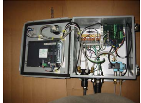
Internal view of screen/PLC enclosure
